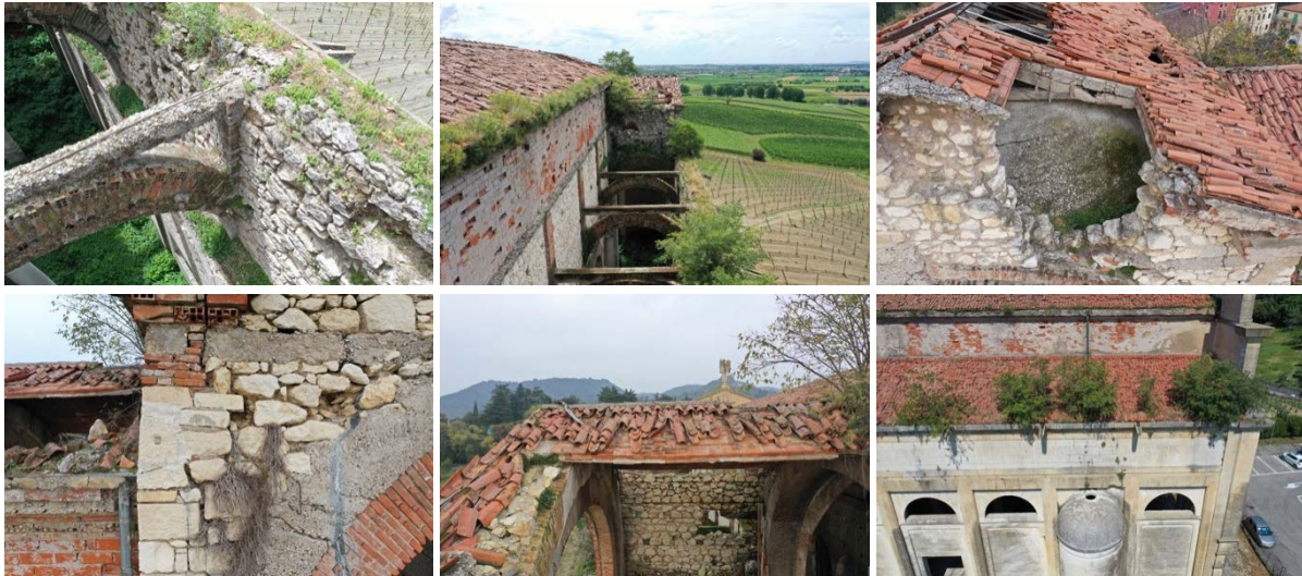
Fig. 5: Some photos referred to the conservation status of the architectural elements of the church.
